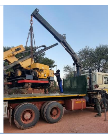
Right: A ramming machine, bought second hand and repaired in Alex' workshop, on its way to the solar plant.
