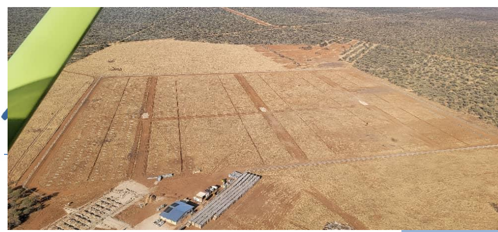
Left: Aerial photo from the plane of the soon-to-be solar plant. The trenches serve to harbour the many electrical cables.
